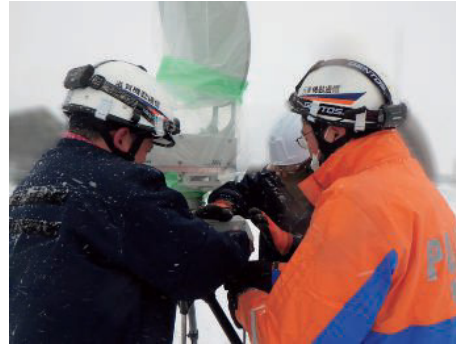
Temporary installation of receiving equipment for a helicopter television system
