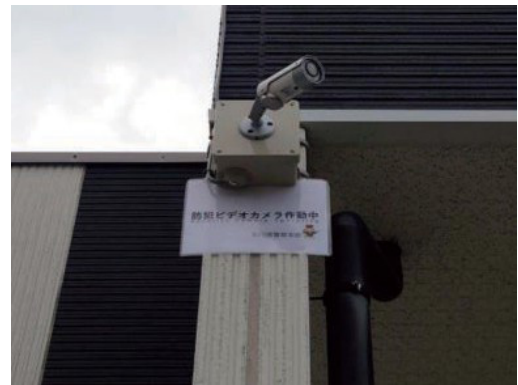
A security camera installed in an affected area
